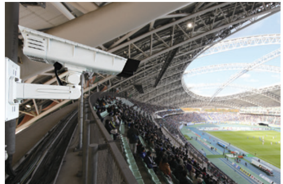
Network cameras used in a stadium
