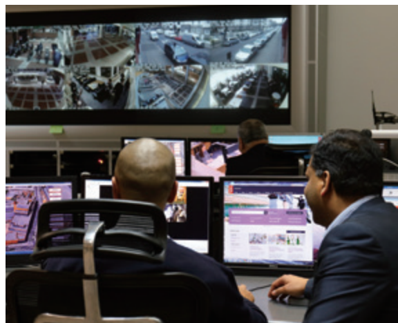
Building monitoring room
