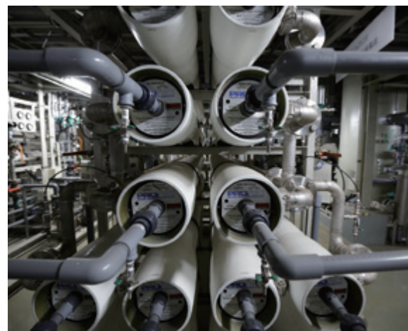
Wastewater filtration system at the Utsunomiya Plant of Canon Inc.
